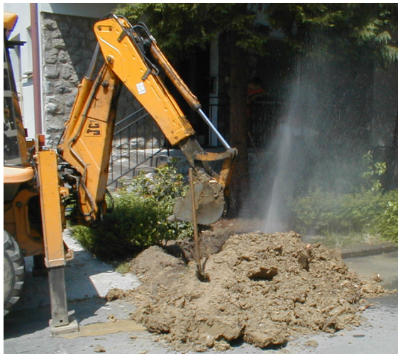
Figure 1 Obvious leakage of pipeline
