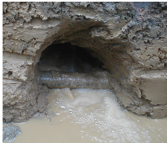
Figure 2 Hidden leakage of pipeline
